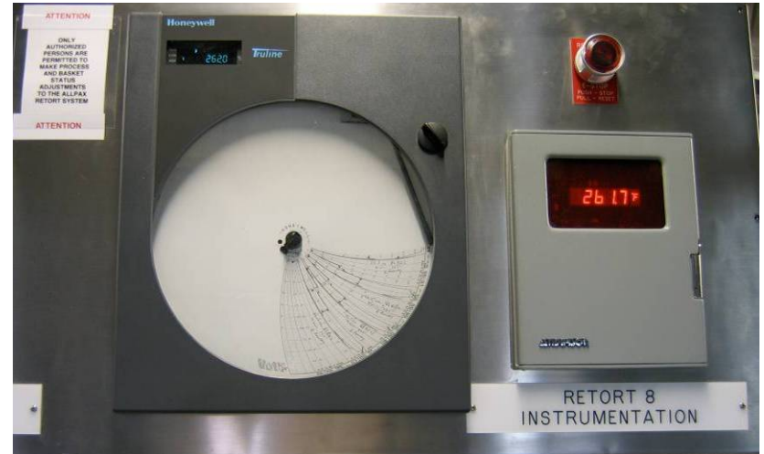
Display mounted remotely on operator deck
