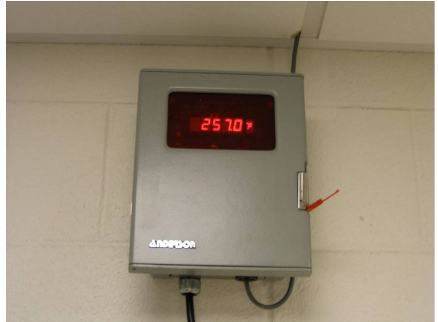
Display mounted remotely in control room
